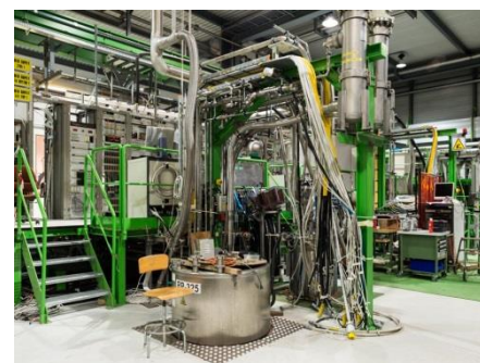
/CERN SM18 Superconducting Magnet Test Facility/
